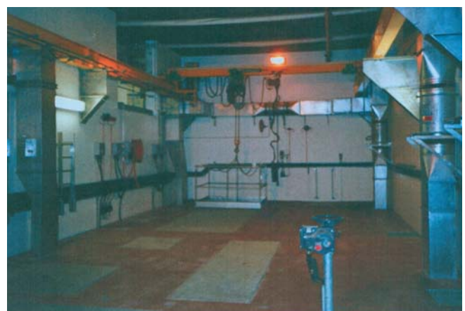
Main hall - pumping station (courtesy Scottish Water)
