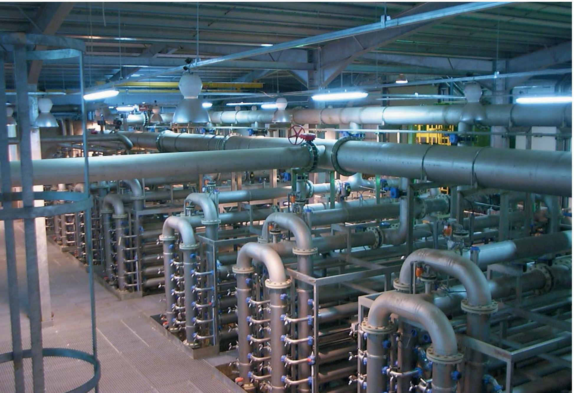
Inveness WTW Membrane skids (courtesy Earth Tech Engineering Ltd)
