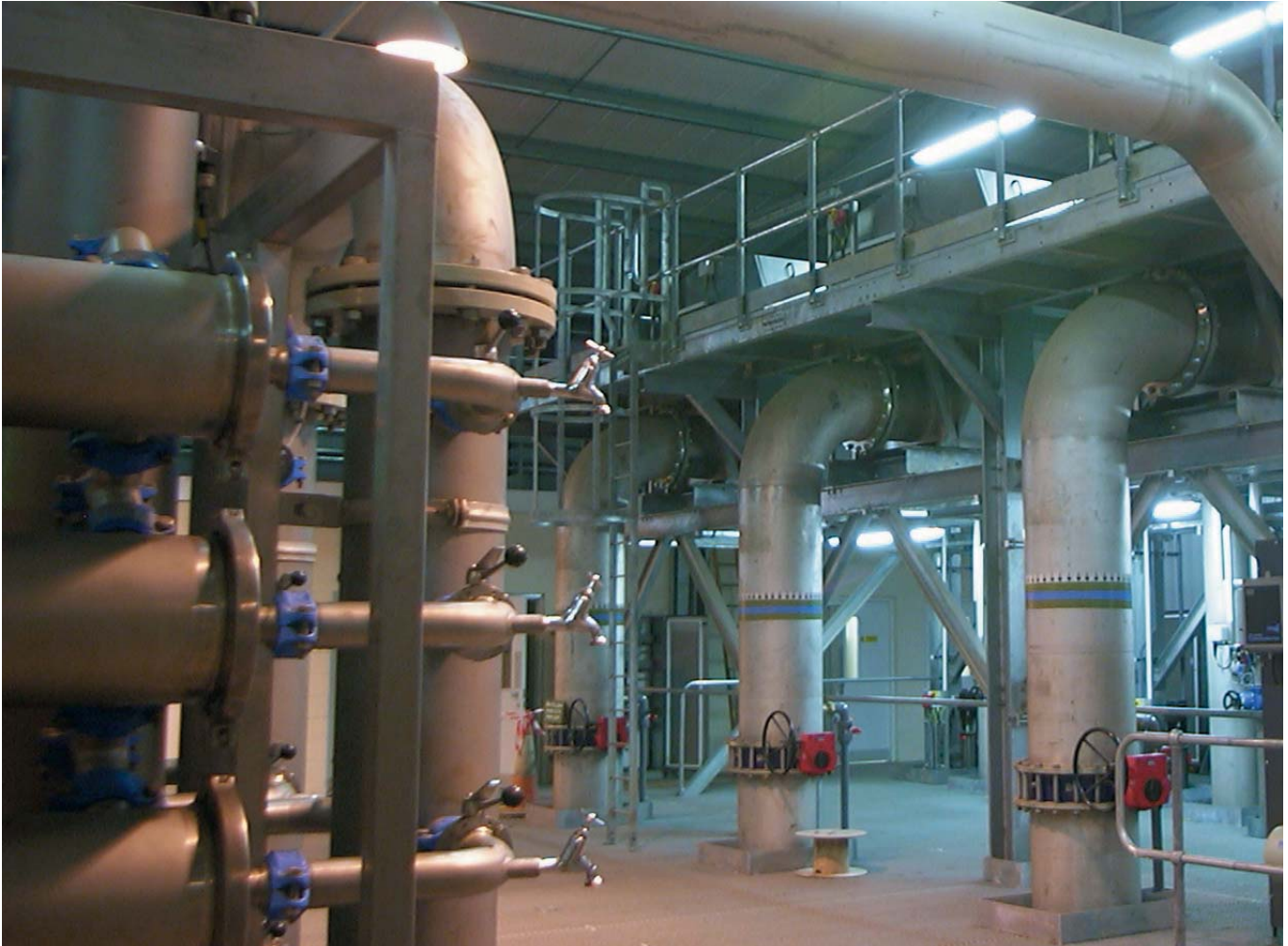
Inverness WTW View of micro-strainers (courtesy Earth Tech Engineering Ltd)
