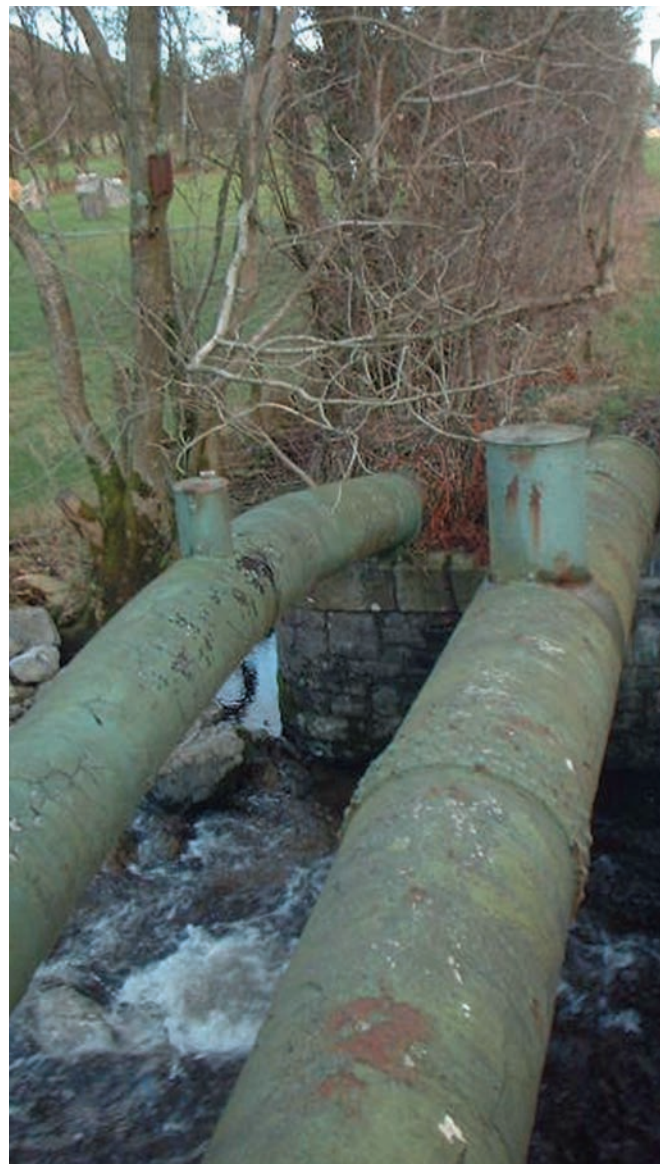
Rehabilitation 100 year old twinned water network trunk main (courtesy Welsh Water Alliance).
