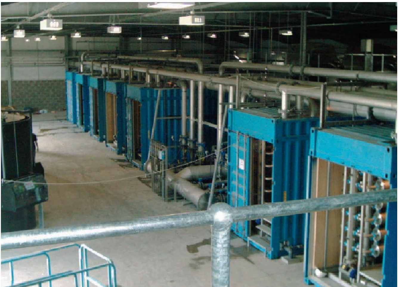
Membrane Plant in six containers
