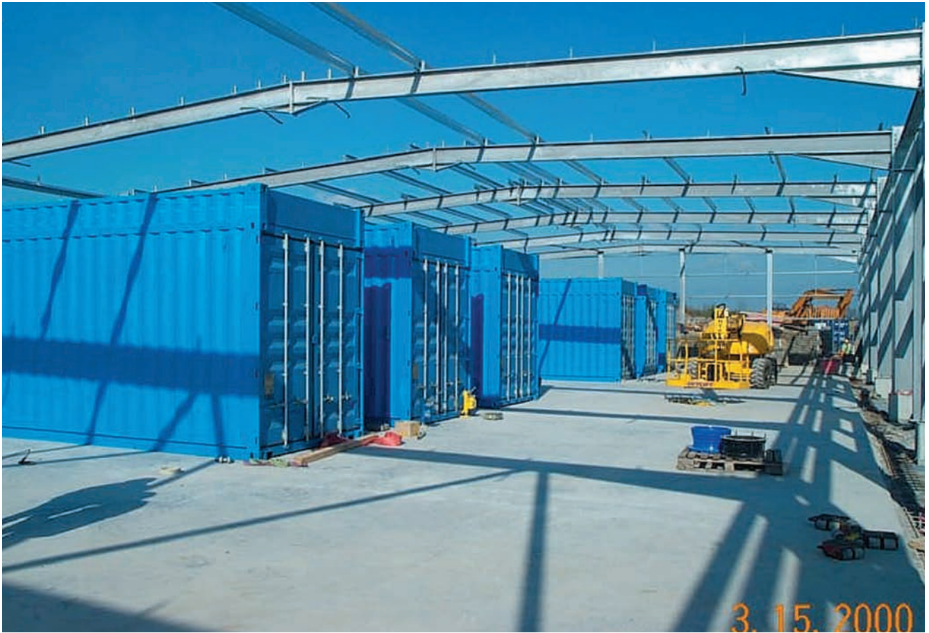
Membrane Plant in six containers
