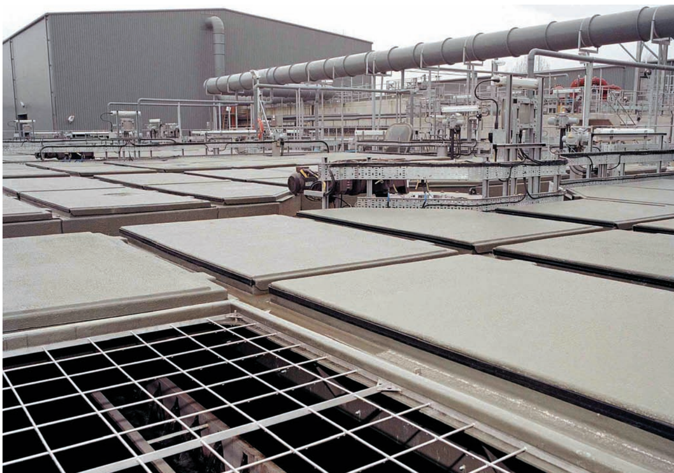
Sandown WwTW – Primary settlement tanks (courtesy Southern Water)
