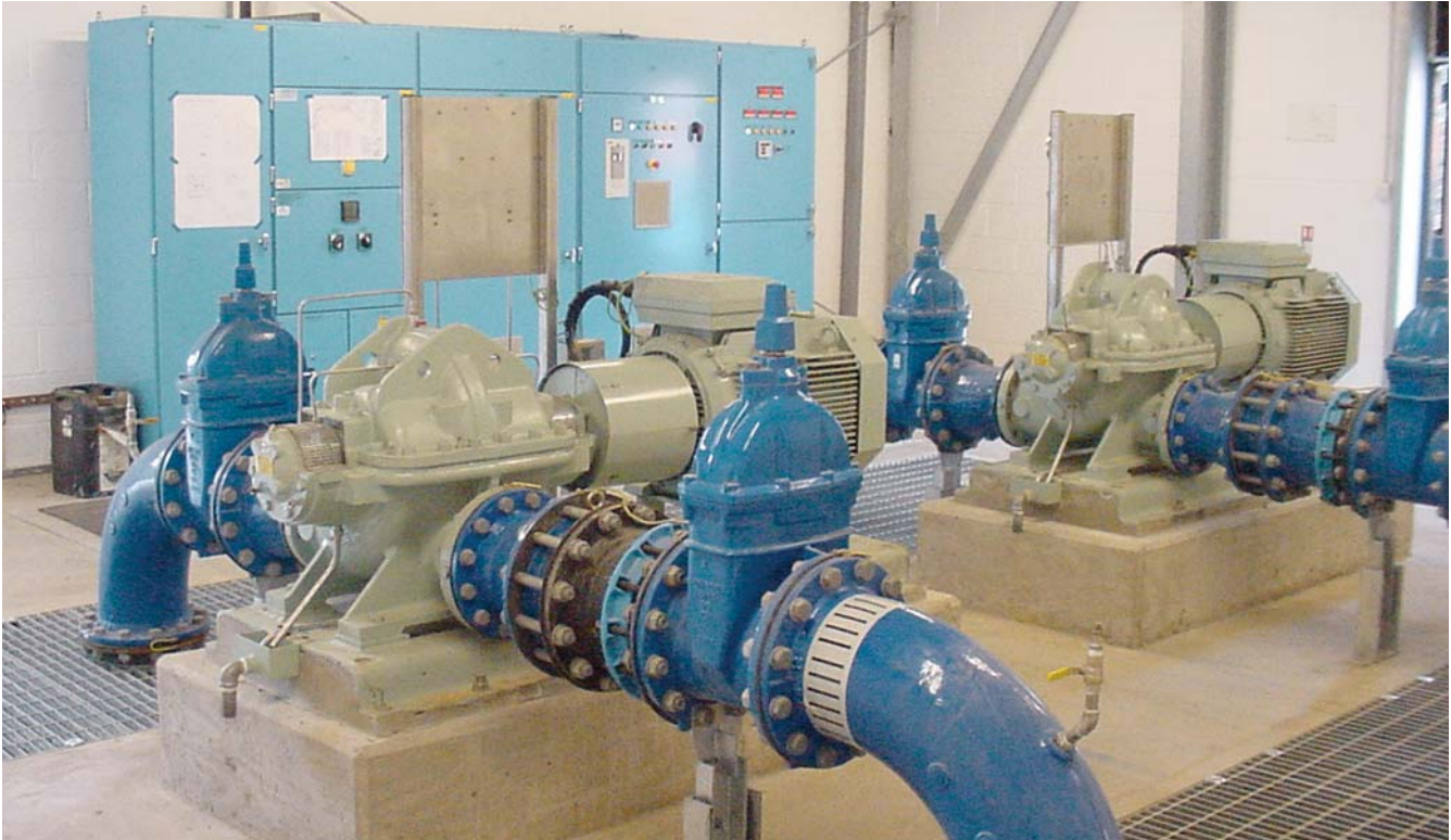
Typical pumping station in three year programme
