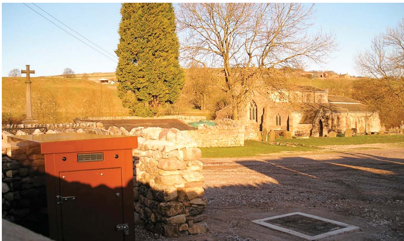
Linton Falls PS: Photo show reinstated car park and pumping station kiosk hidden by stone wall
