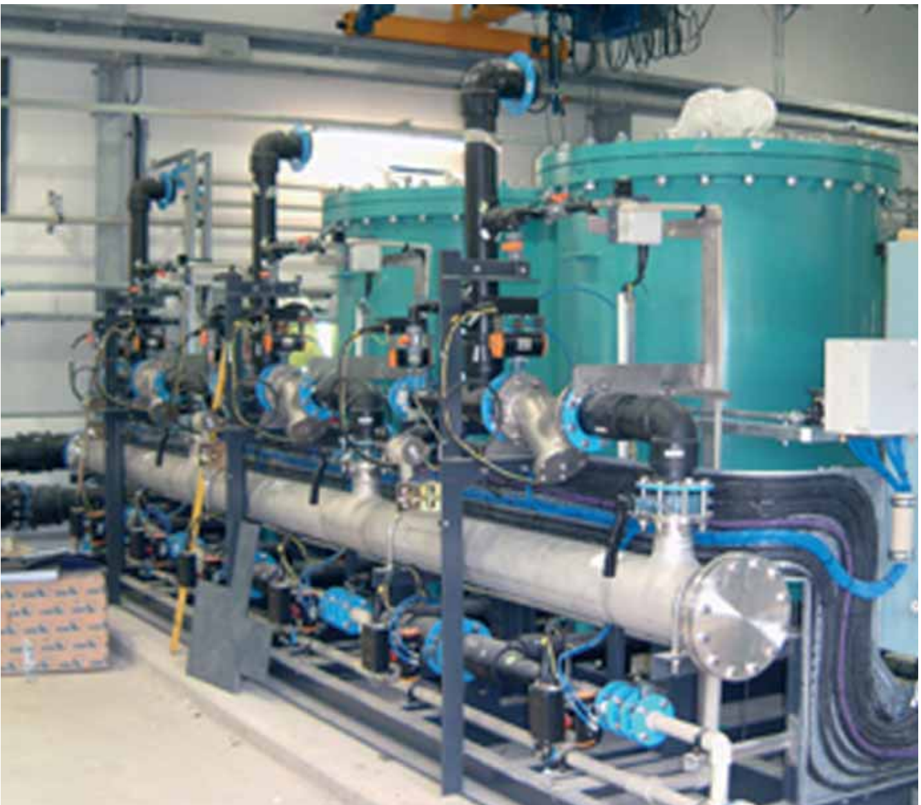
Clarendon Nitrate Reduction Scheme: Anion Skid inside new process building
