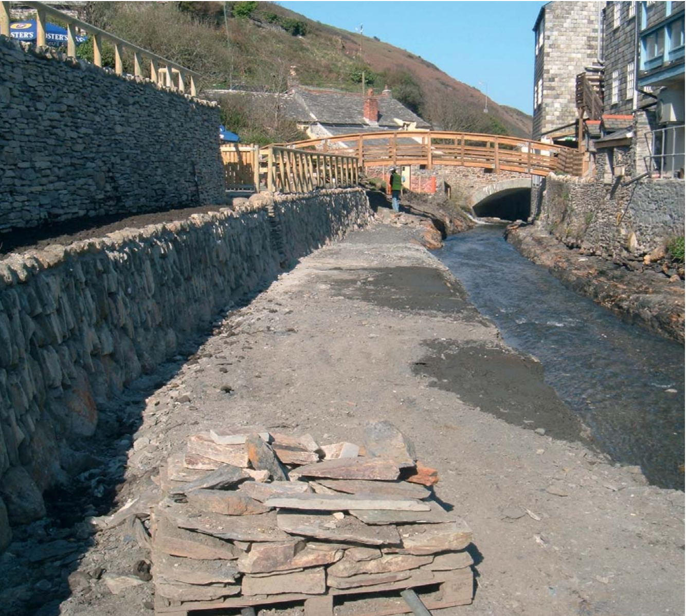
Photograph shows the channel after widening & deepening, part of the Environment Agency's £4million Flood Defence Scheme
