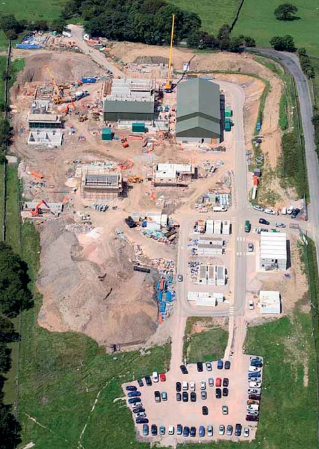
Clean backwash pumps flanked by second stage filters and chemical building with admin building in the distance.
