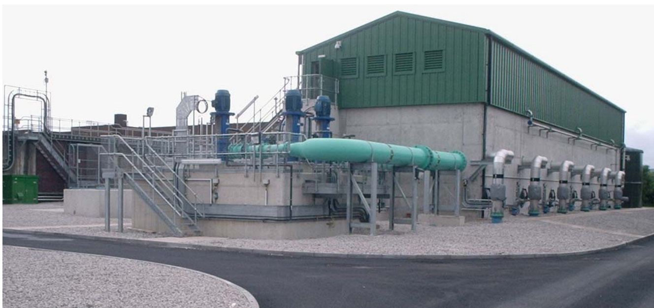
Bretton Water Treatment Works GAC Plant
