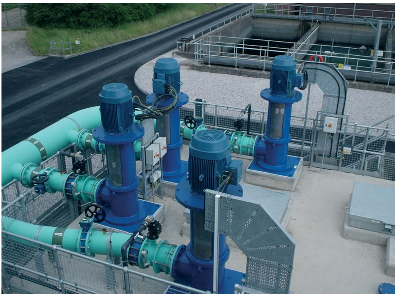
Bretton Water Treatment Works GAC plant
