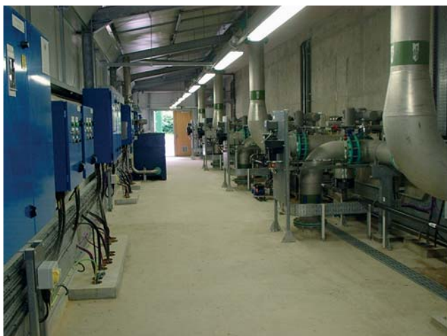
Bretton Water Treatment Works GAC Plant
