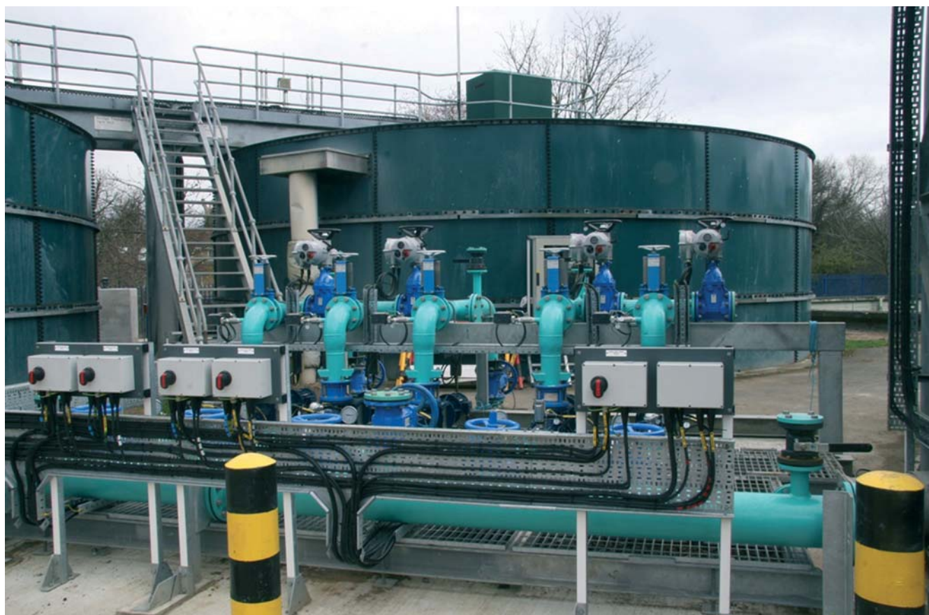
New Thickened Sludge Transfer Pump skid. Existing WRc Thickener in background
