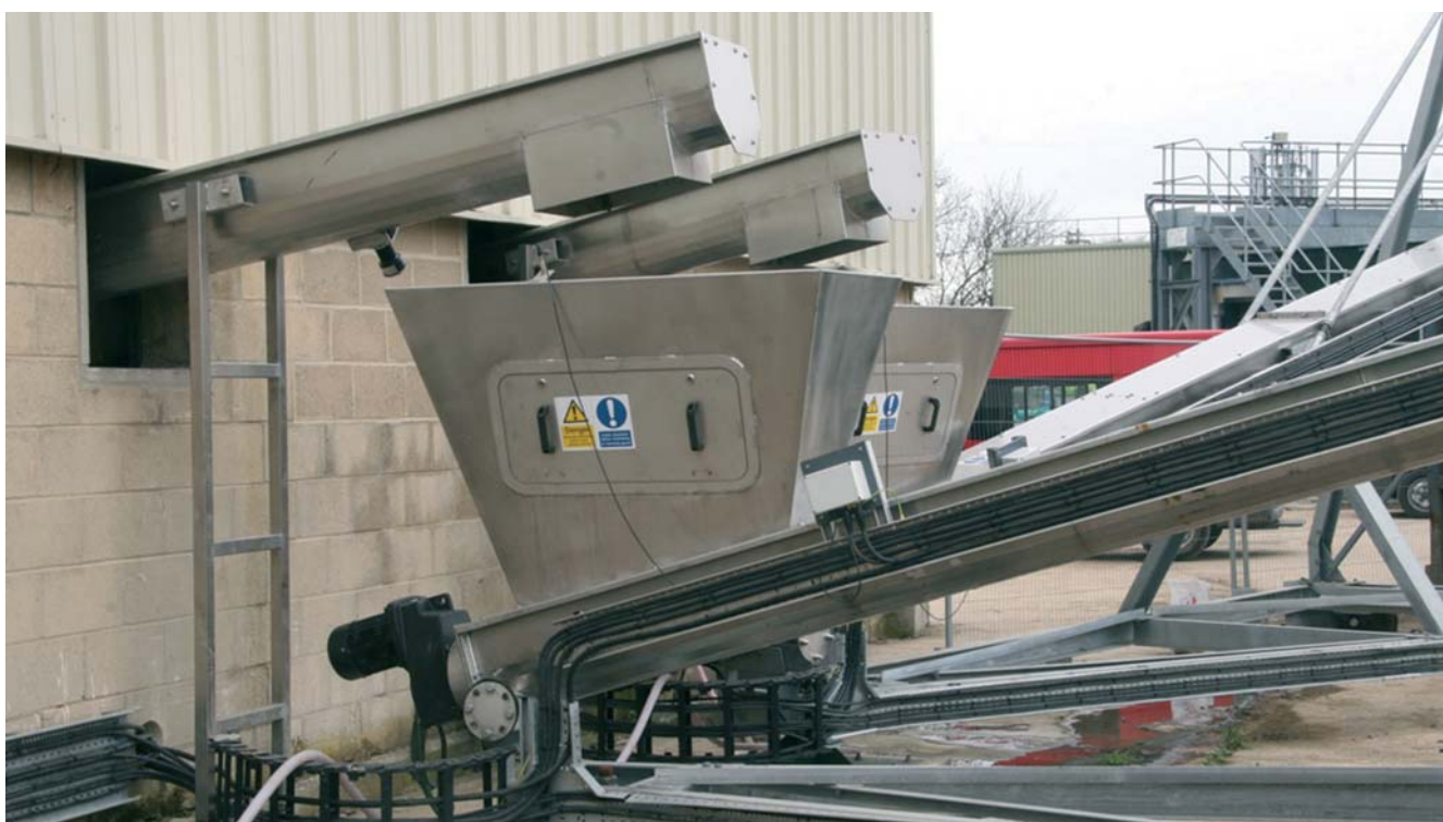
Horizontal Screw Conveyors feeding external hoppers for the inclined Conveyor system
