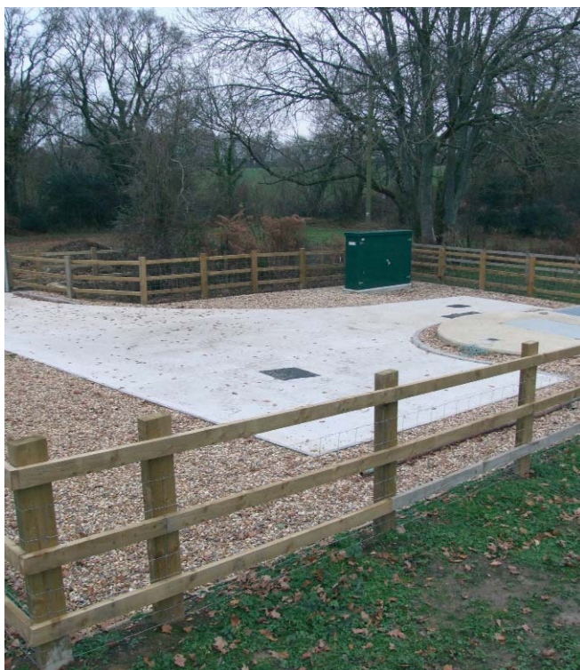
Bussons Corner pumping station in Holt Village
