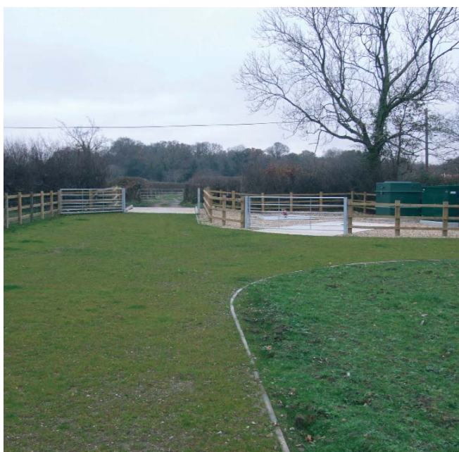
Holt Vale pumping station in Holt Village
