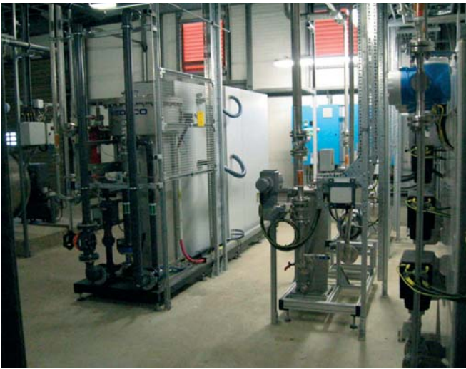
New CODs and ozone generator (left) and Wedeco SMO 600S unit (right)
