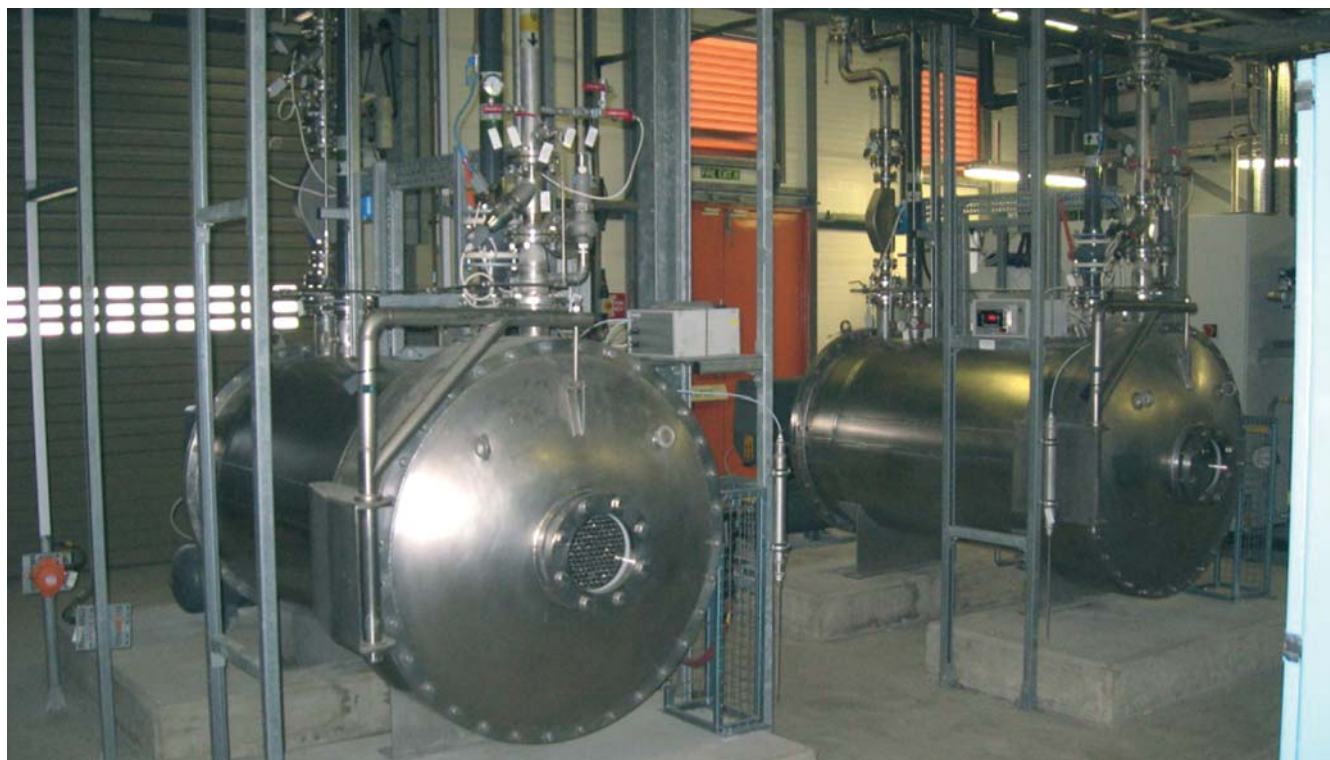
Existing ozone generators
