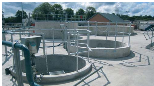
Flow metering chambers with one of the primary settlement tanks in the background
